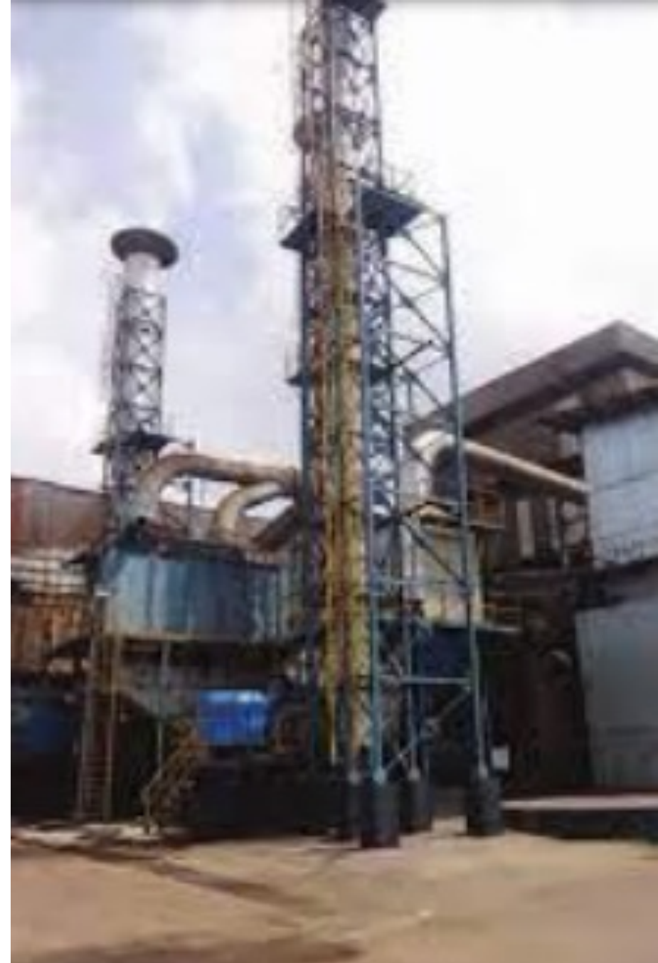
Power Plant – 40 MW
