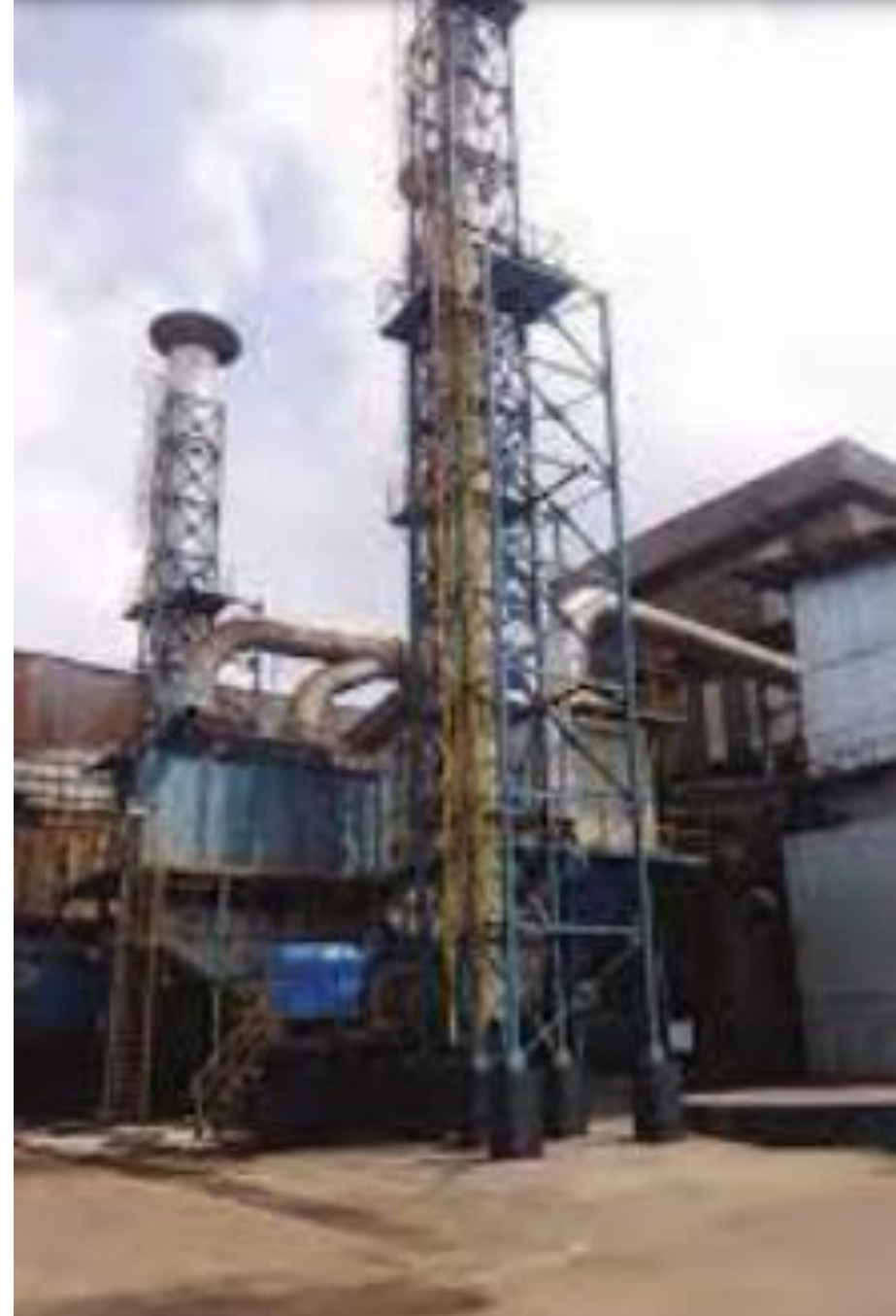
Power Plant – 40 MW
