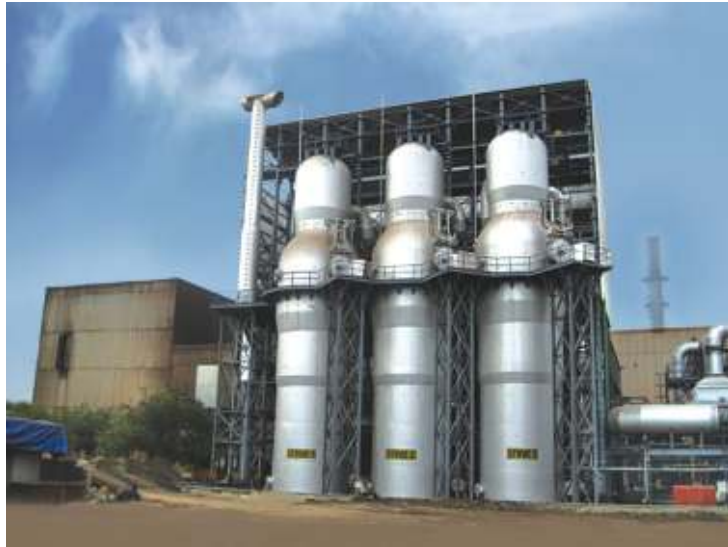
Installation of hot blast stoves for second mini blast furnace at Bevinahalli.
